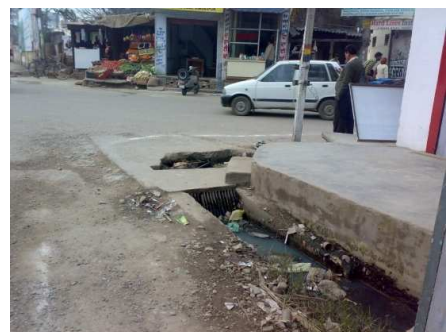
Fig no. 37: Blocked Sewerage at P.O. Chowk
