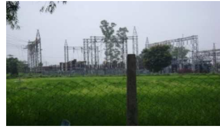
Fig no.42: 132 KV Grid station at Hardo Channi Road
