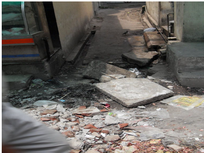
OPEN DRAIN, NO SEWERAGE
